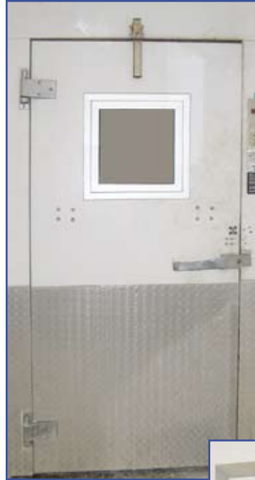
Damaged doors like the one at left place stored product at risk.
