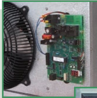
The Master Controller panel (shown above with housing removed) is mounted to the evaporator.
