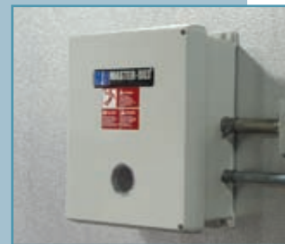
Other boards for plasma and storage freezers are mounted on the outside of the walk-in in a protective housing.
