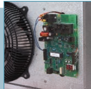
One Master Controller Reverse Cycle Defrost board (shown with cover off) is mounted to the evaporator coil in the ante-room.
